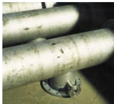
Fabricated pipe showing carbon steel pickup.
