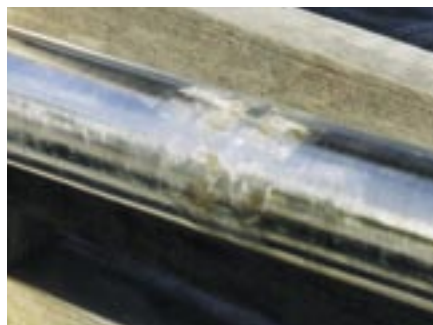
Corrosion on a handrail caused by rough grinding.
