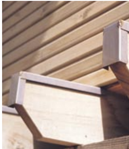
Scale on a welding site. Note the crevice corrosion and corrosion from the weld heat tint at this seaside site.
