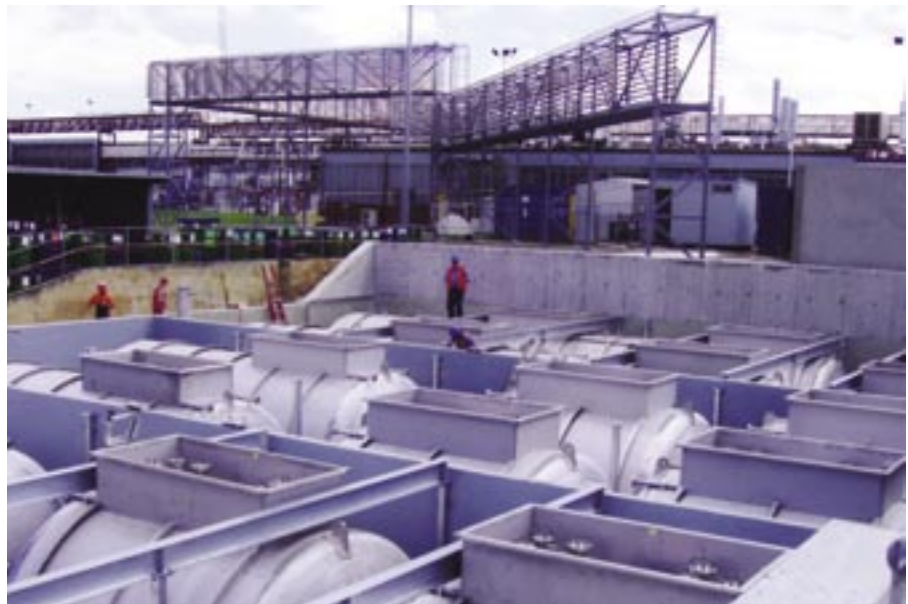
The Bulk Solvent Storage (UST) project at PPG Industries Australia, Clayton site includes multiple stainless steel bulk storage tanks contained within a concrete vault. Below: Furphy Engineering at Shepparton undertook the construction together with a substantial volume of stainless pipe spool work.
