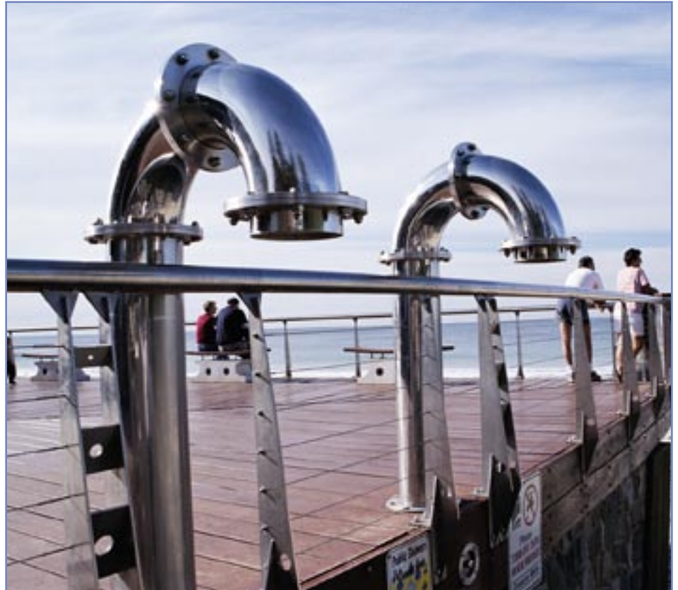
ABOVE: A successful stainless steel installation in a coastal application, with no tea staining.
