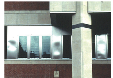
Buckling caused by insufficient allowance for solar heating.
