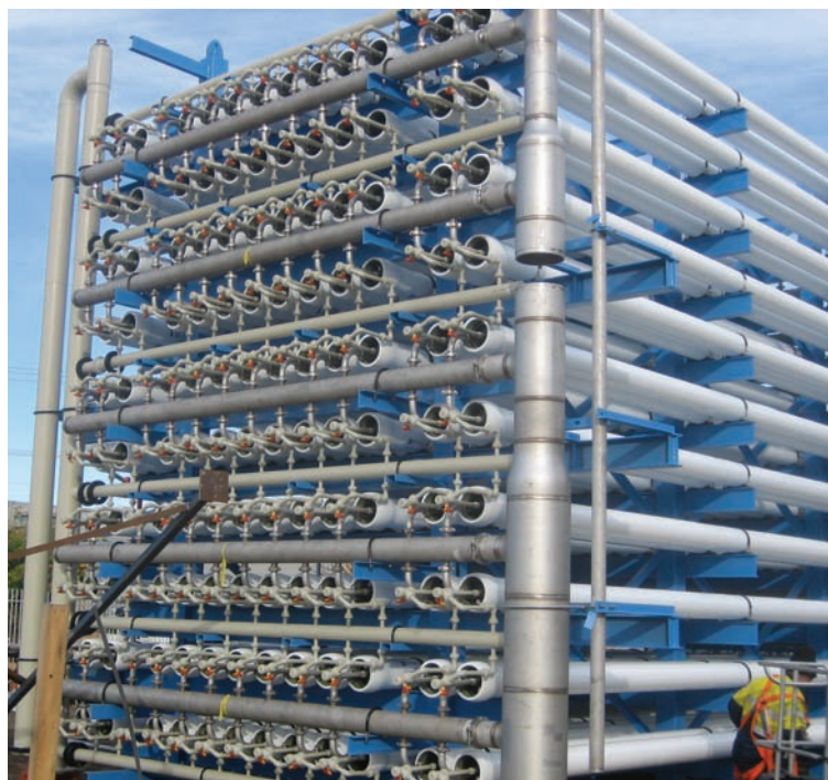
Reverse osmosis racks
